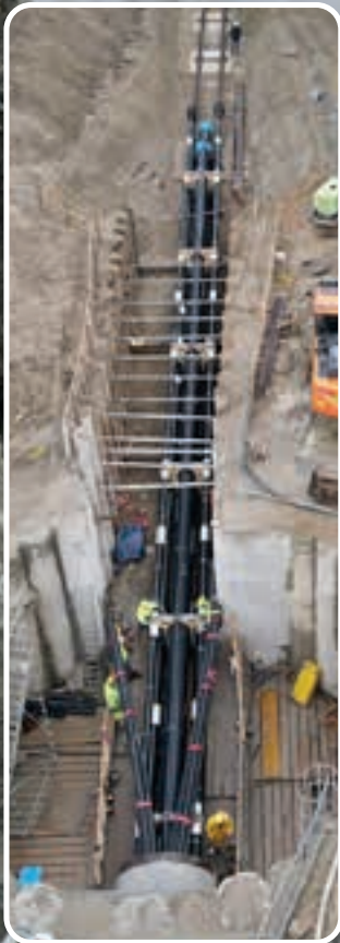
Siphon under the Danube, laying pipelines for drinking water, district heating, fiber optics, and gas.
